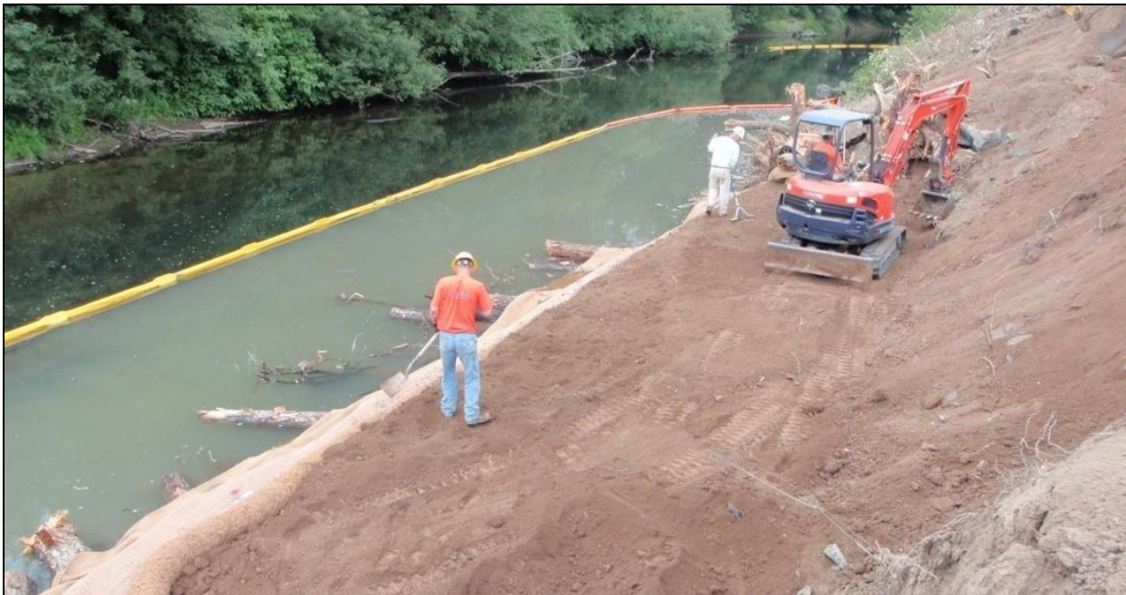
Figure 5-2. Example of a silt curtain isolating an active work area from clean water flowing by the project site. Turbid water is contained within the work area by the silt curtain.
