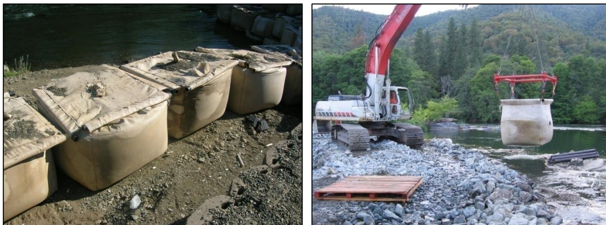
Figure 5-1. Example of bulk bags (left) used for work area isolation and moving a loaded bulk bag (right).
